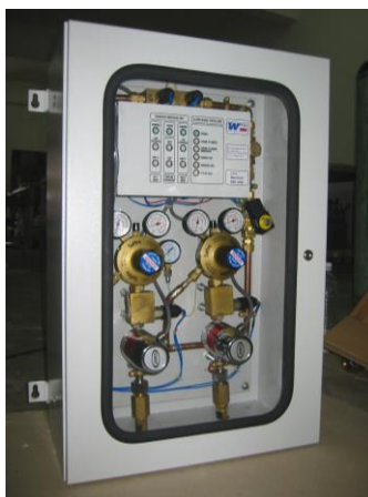
Autochangeover panel with heater
